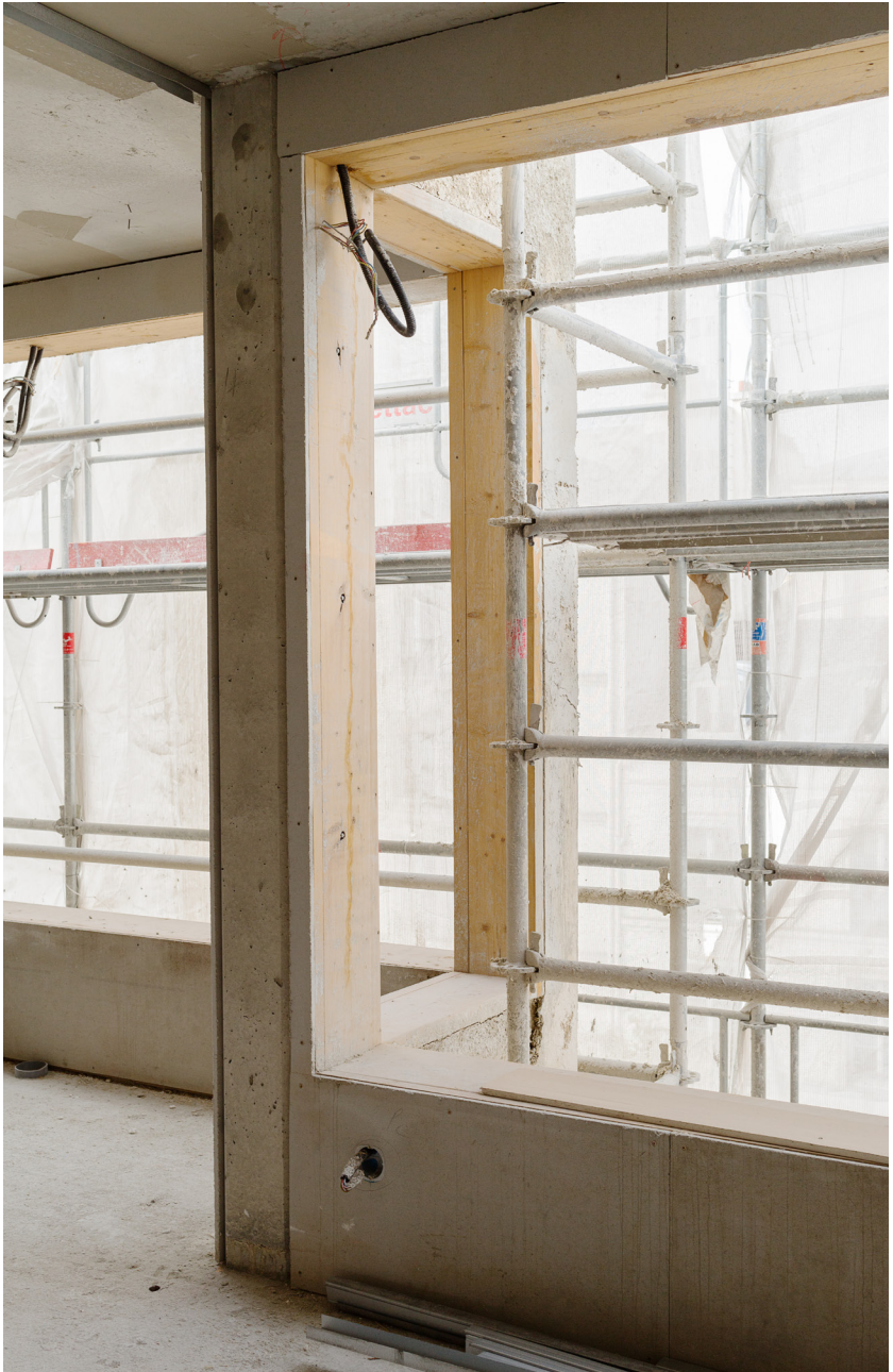
Fig. 2 - The hempcrete is the whole envelop of the building. The insulation is the whole wall.
